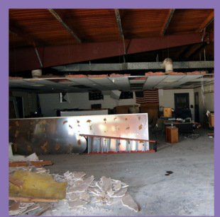
The storage area in the Ag Shop, adjacent to Mr. Almquist's classroom, was removed to make room for classrooms.
